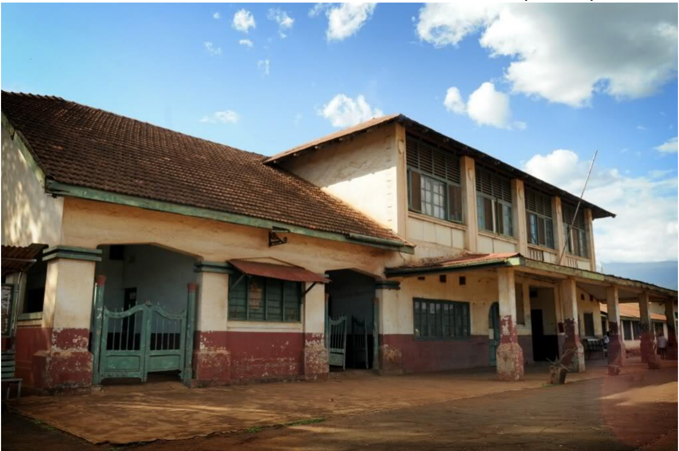
Moshi Railway Station in a depleted state and hardly operational except for two or three freight trains a week. (Recent)
